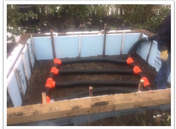
Installation of a thermal rock bed in a home passive solar greenhouse. Image by Kim Ross, University of Saskatchewan.
